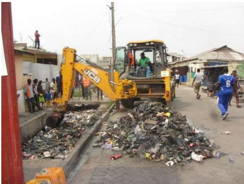
Figure 1.3 Garbage in an open drain in Accra
